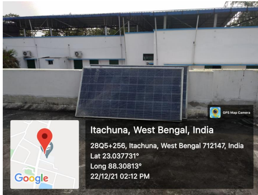
Solar Panel in Bejoy Narayan Mahavidyalaya
